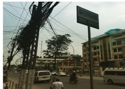
Figure 20. A dangerous and complicated power wires system in Kathmandu
