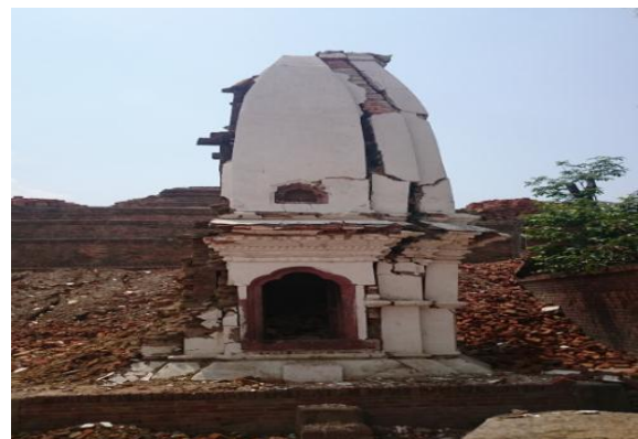
Figure 6. Destroyed historic monuments at Durbar Square of Bhaktapur.
